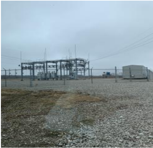
Photo 25. Photo of Duke electrical systems.
