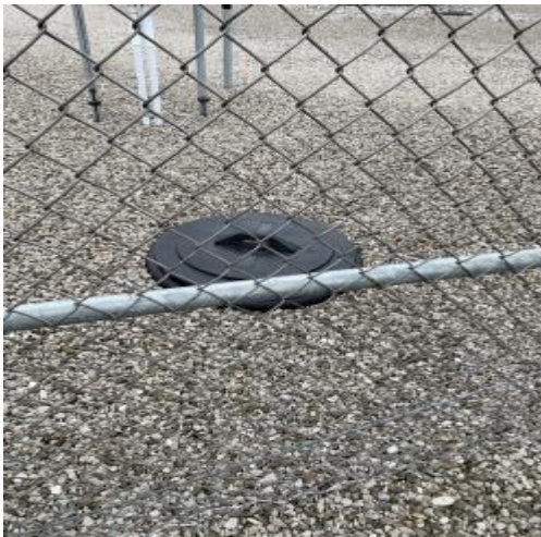
Photo 27. Photo of Duke Energy electrical systems.
