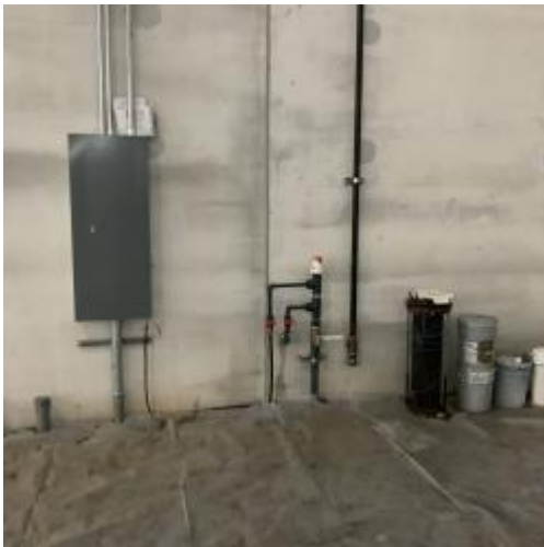
Photo 11. Photo of utilities.
