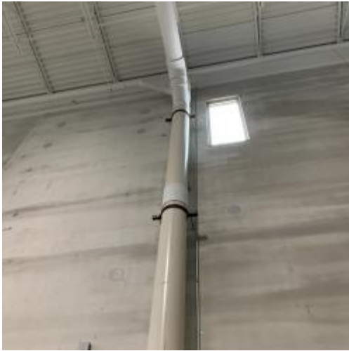
Photo 13. Photo of interior piping.
