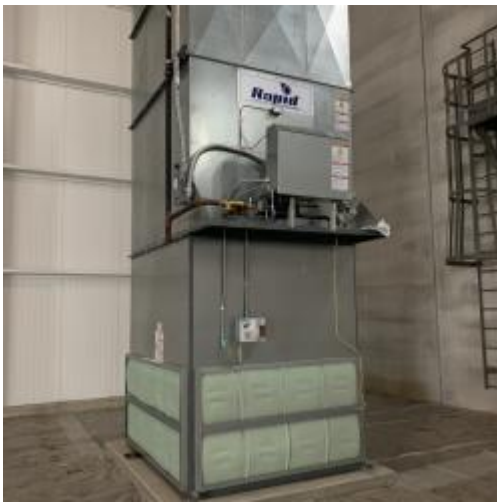
Photo 9. Photo of HVAC systems.
