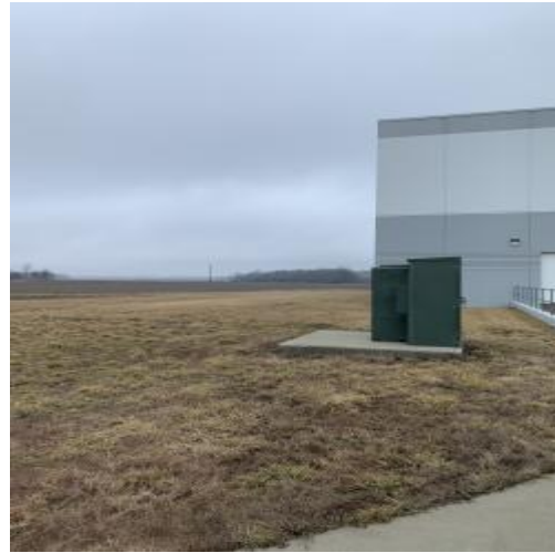
Photo 14. Photo of transformer.
