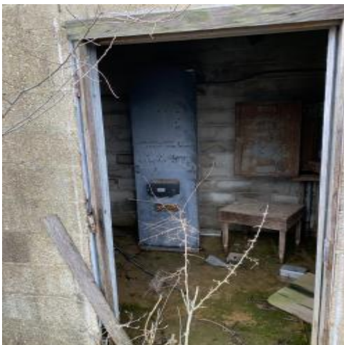
Photo 29. Photo of electrical outbuilding.
